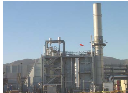
Rentech HRSG with SCR and duct firing.
