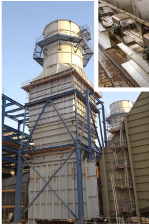
Bypass Dampers, Silencers and Stacks
