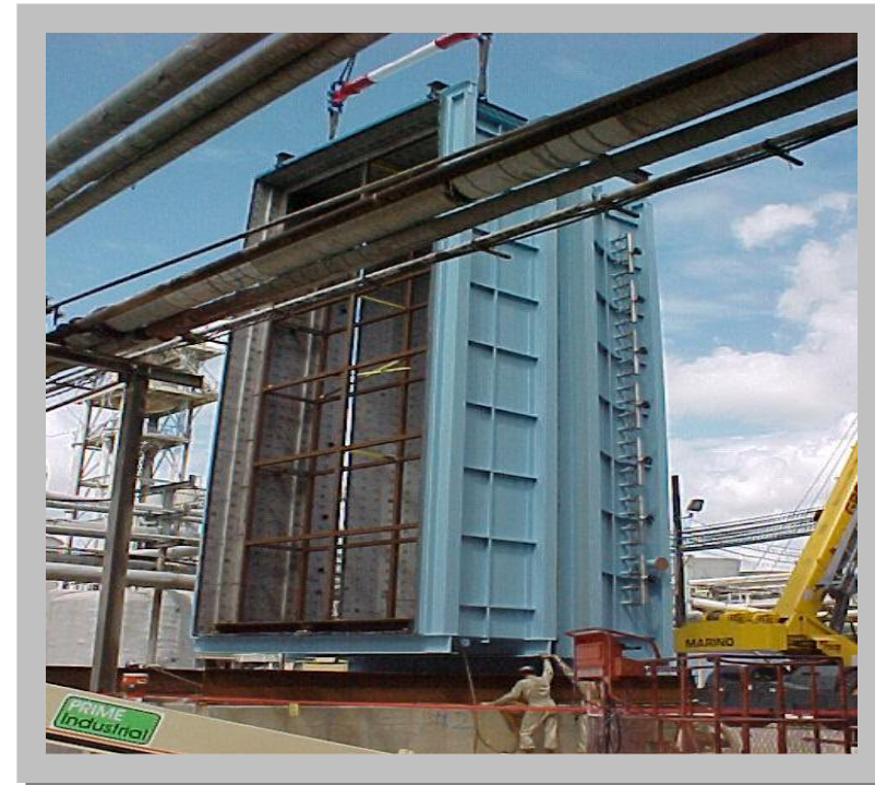
SCR Retrofit for Gulf Coast Refinery Cogen
