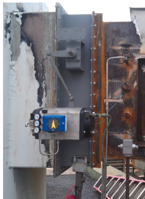
New Boiler #1 Draft Damper
