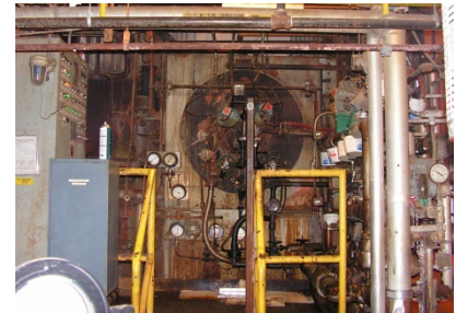
Boiler #1 Burner before retrofit
