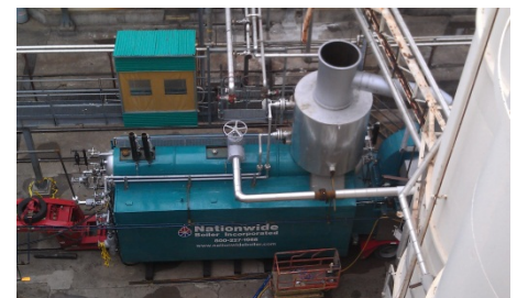
75,000 PPH Rental Boiler
